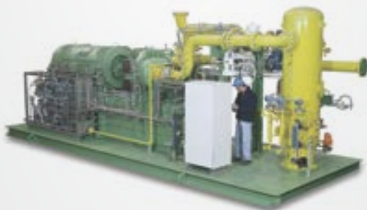
Fuel Gas Booster Skid
